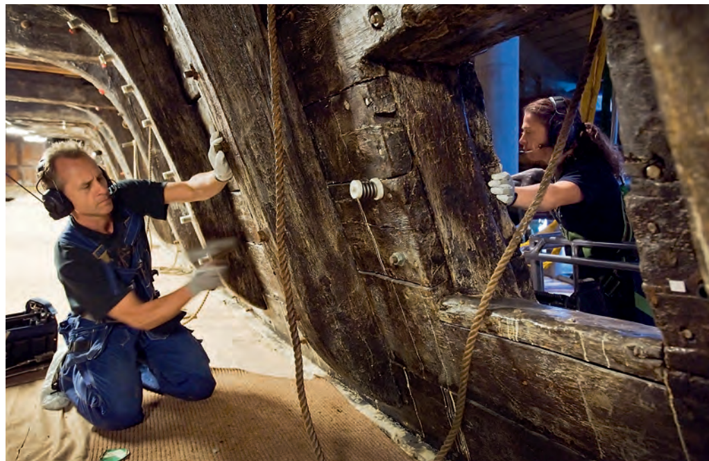
Varying hole sizes and amounts of corrosion demand that individual attention be given to each bolt. © Anneli Karlsson, the Swedish National Maritime Museums
