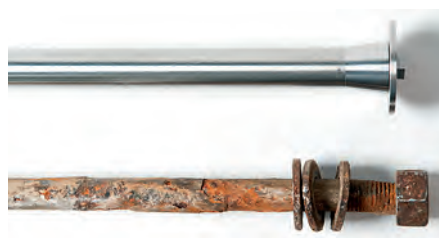
The old rusting mild steel bolts are replaced one by one with new super duplex stainless steel bolts. © Anneli Karlsson, the Swedish National Maritime Museums
